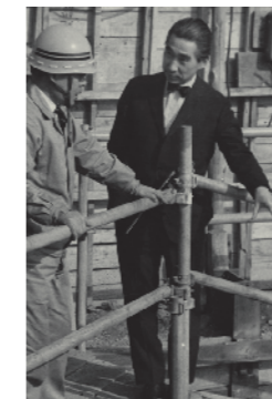
建築中に現場を見てまわる丹下健三氏。 Kenzo Tange visiting the site during construction
