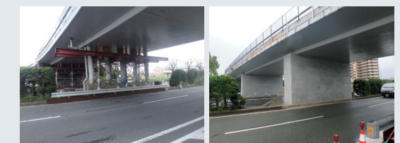
Higashibarū Bridge (Kumamoto Prefecture) emergency restoration underway (left) and after seismic reinforcement (right)
