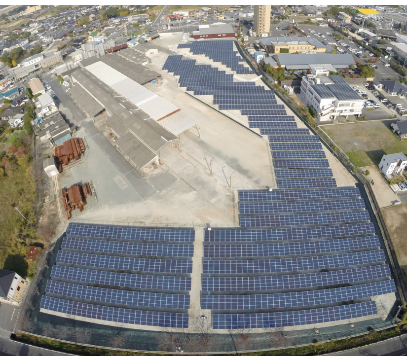
Mitagawa Solar Power Plant
