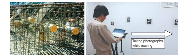
Sleeves for pipework
