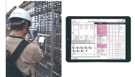
Equip tablet terminals with execution management functions to inspect bar arrangement, take photographs of bar arrangement, etc.
