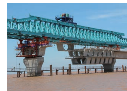
Lach Huyen International Port construction (road and bridge) using precast segment span-by-span method
